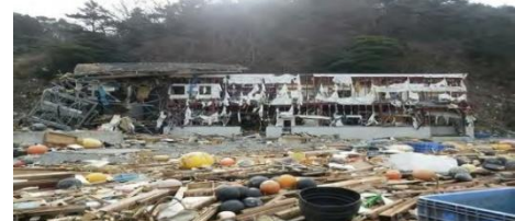
Fish processing facility at Yoriiso Port damaged by tsunami (Ishinomaki, Miyagi Pref.)
